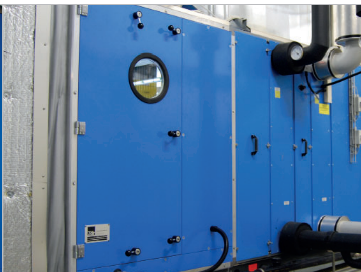
7Air revision front mounted on humidifier section
